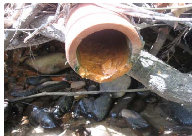
Outfall pipes such as this one can carry pollutants, if they are inappropriately and illegally dumped, directly to our streams.
